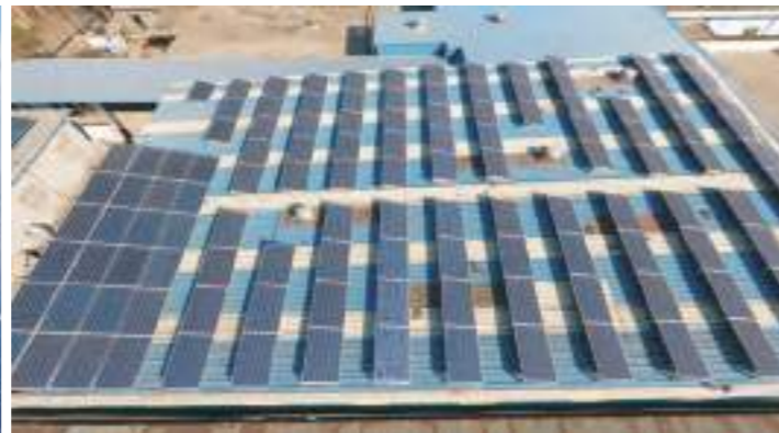
250kw tilt solution in Thailand
