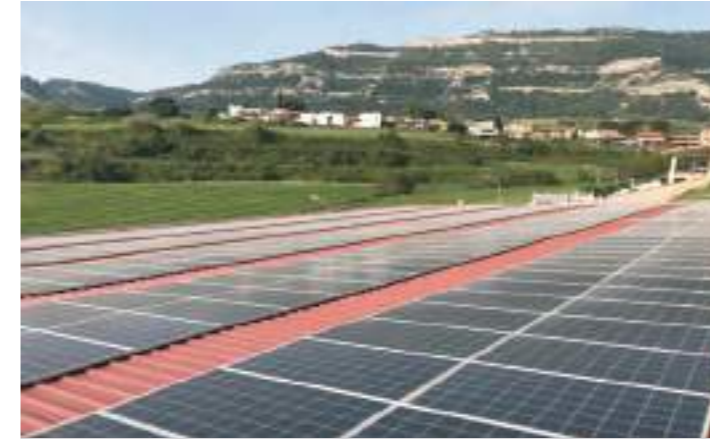
700kw L foot solution in UK
