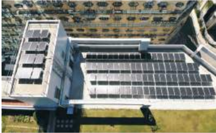
200kw flat roof solution in Hongkong
