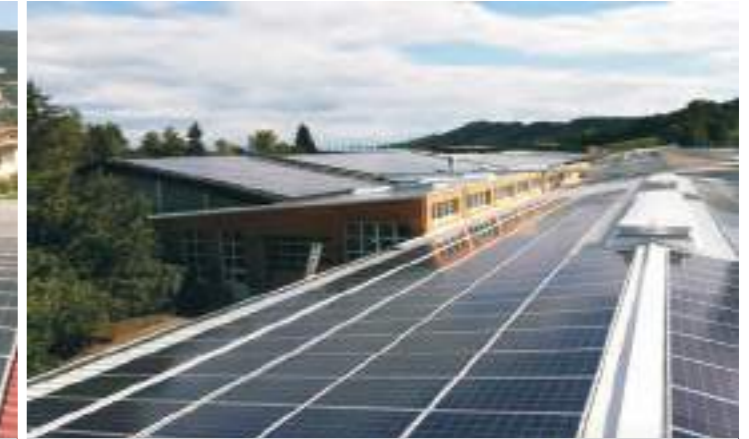
2.4mw railless solution in New Zealand
