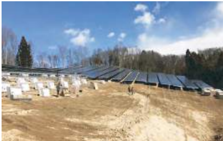
3.8mw sloping mounting solution in Japan
